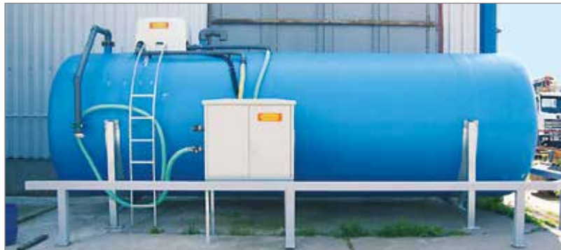
Completely installed brine unit including pump
