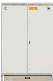
Closed with warning signs
